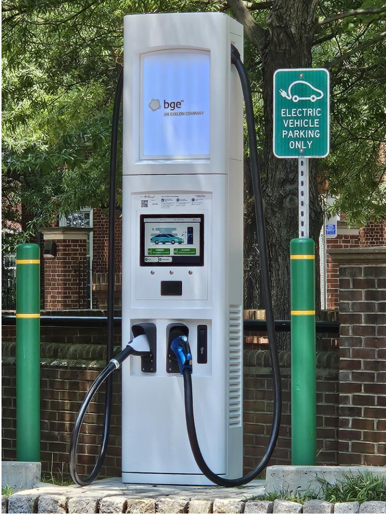
Electric Vehicle Chargers Ribbon Cutting on June 17
