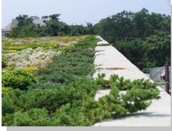
Green Roof on Severn Savings Bank Courtesy of: O'Doherty Group Landscape Architecture
