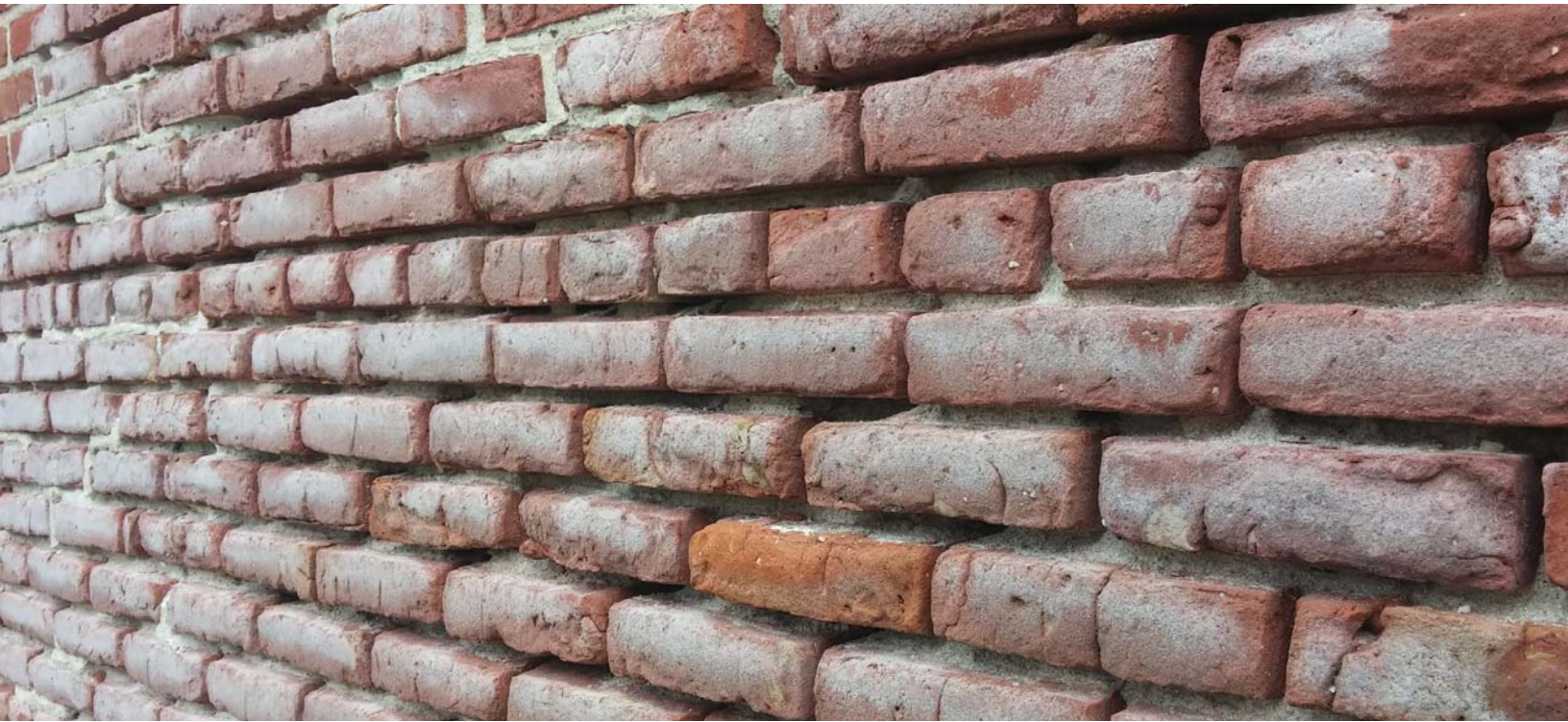
Effects of Hurricane Sandy on masonry in Crisfield, MD Photo credit: Lisa Craig
