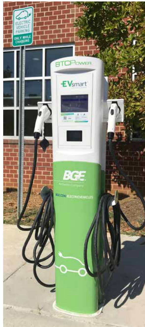
FIGURE 9-28: EV CHARGER AT PIP MOYER RECREATION CENTER
