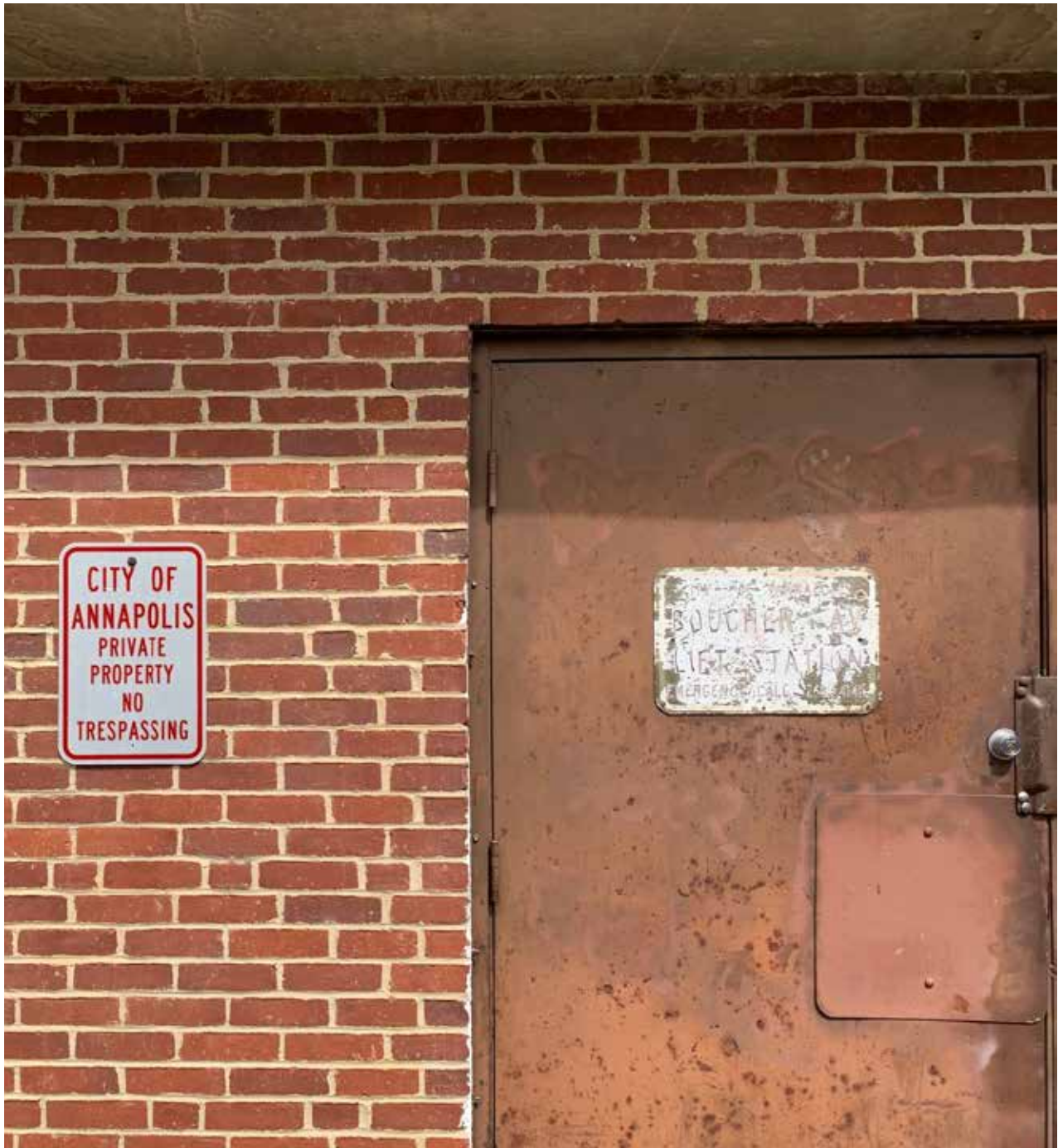
FIGURE 10-16: THE CITY'S BOUCHER AVENUE LIFT STATION LOCATED AT HAWKINS COVE IS ONE OF MANY SMALL BRICK STRUCTURES LOCATED THROUGHOUT THE CITY THAT HOUSE PUMPS FOR MOVING WASTEWATER FROM LOWER TO HIGHER ELEVATIONS.
