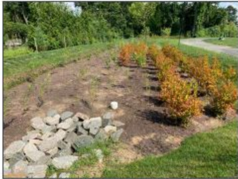
Bioretention facility SOURCE: CITY OF ALEXANDRIA
