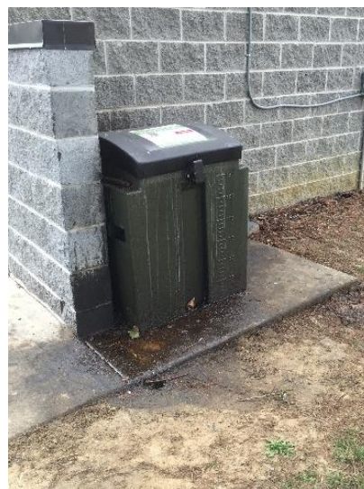
Figure 13. HSI-06a - Grease Storage
