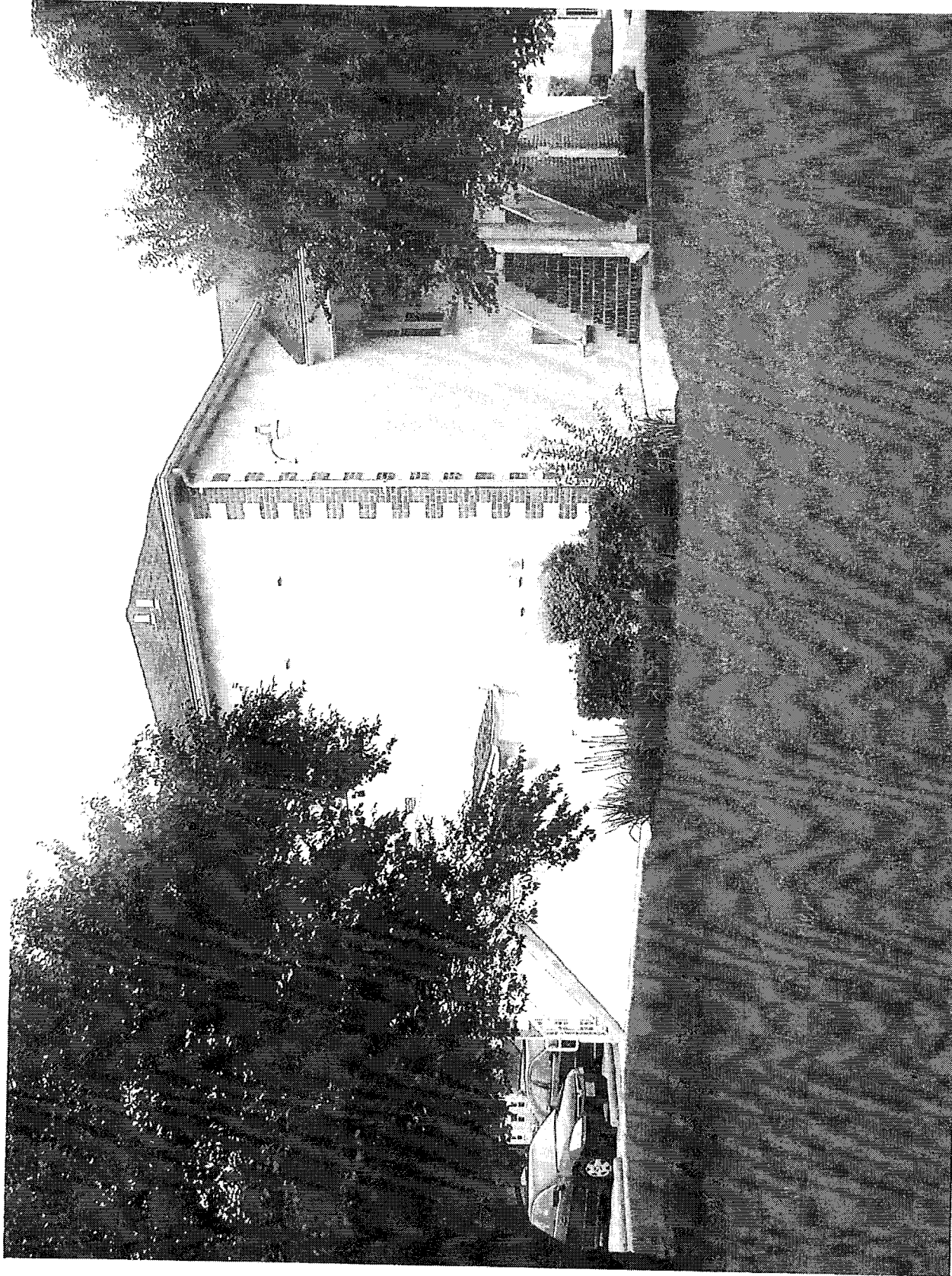
Community Health Center at Parole, Exterior View of Corner of Original Building as Modified, Showing Original Quoins, Looking NE
