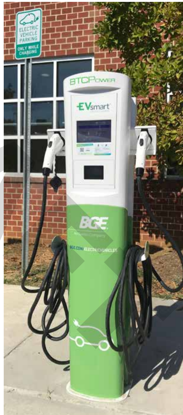
FIGURE 9-28: EV CHARGER AT PIP MOYER RECREATION CENTER
