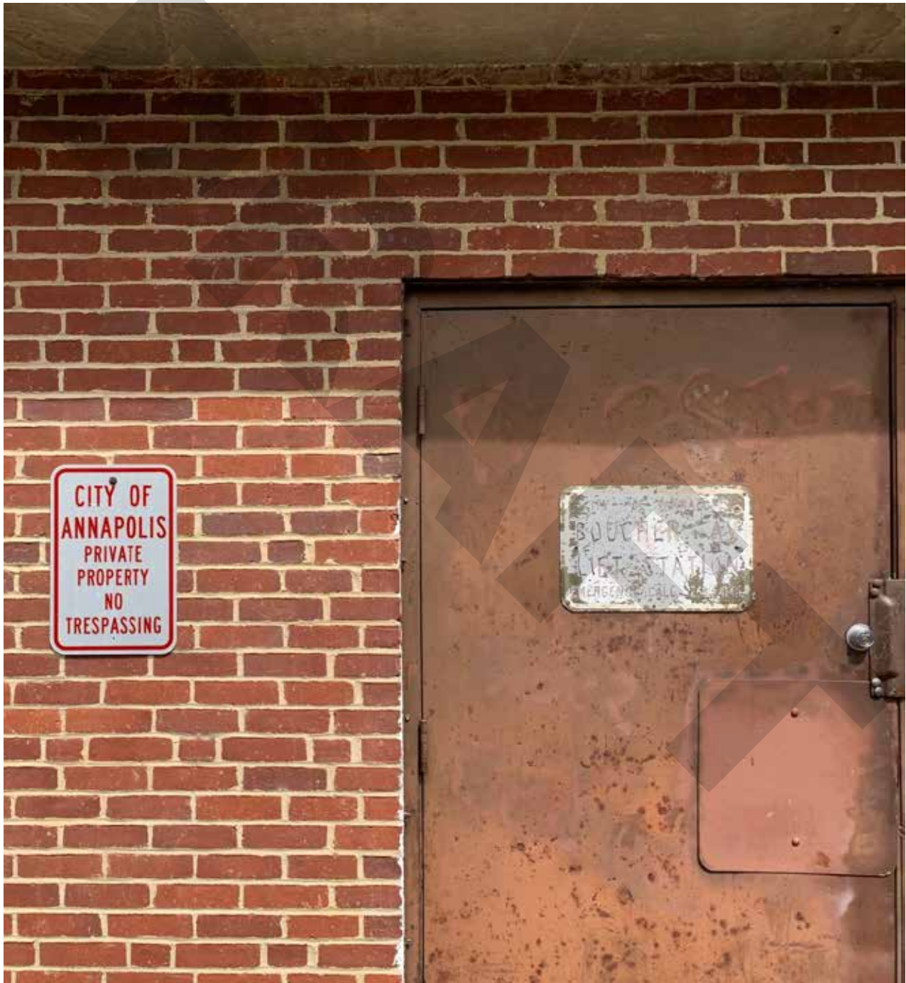
FIGURE 10-16: THE CITY'S BOUCHER AVENUE LIFT STATION LOCATED AT HAWKINS COVE IS ONE OF MANY SMALL BRICK STRUCTURES LOCATED THROUGHOUT THE CITY THAT HOUSE PUMPS FOR MOVING WASTEWATER FROM LOWER TO HIGHER ELEVATIONS.
